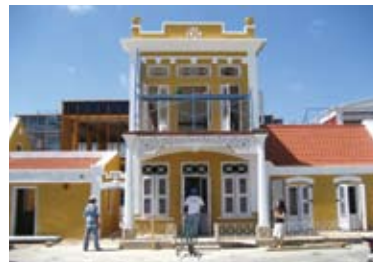
Construction of the new building for the National Archaeological Museum of Aruba.
